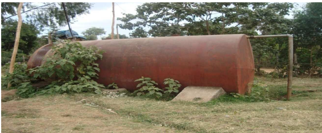
Figure 5: The steel wet well at booster station
