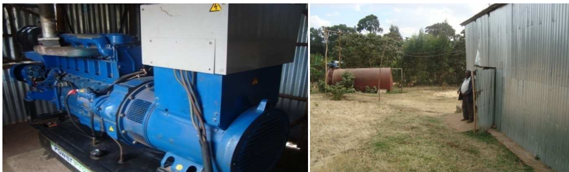
Figure 2: Generator at Gocho Bore hole
