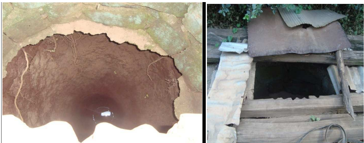
Figure 6: Hand dug well with no proper construction at lalo kebele
