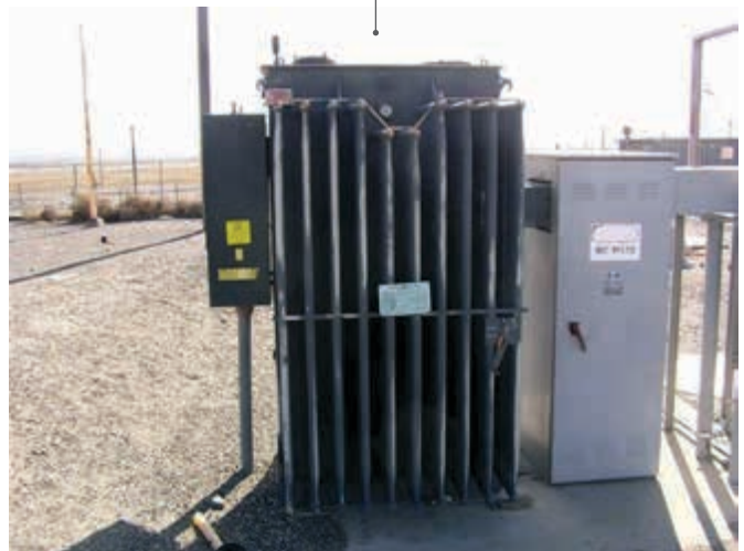
The last PCB-contaminated transformer on the Hanford Site was safely removed and disposed of at the end of September.
