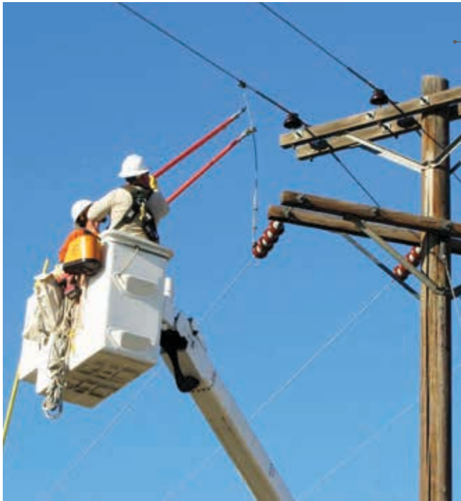
EU linemen Phillip Doras and Nathan Case work on removing jumpers to de-energize power from the line in preparation for the removal of the transformer.
