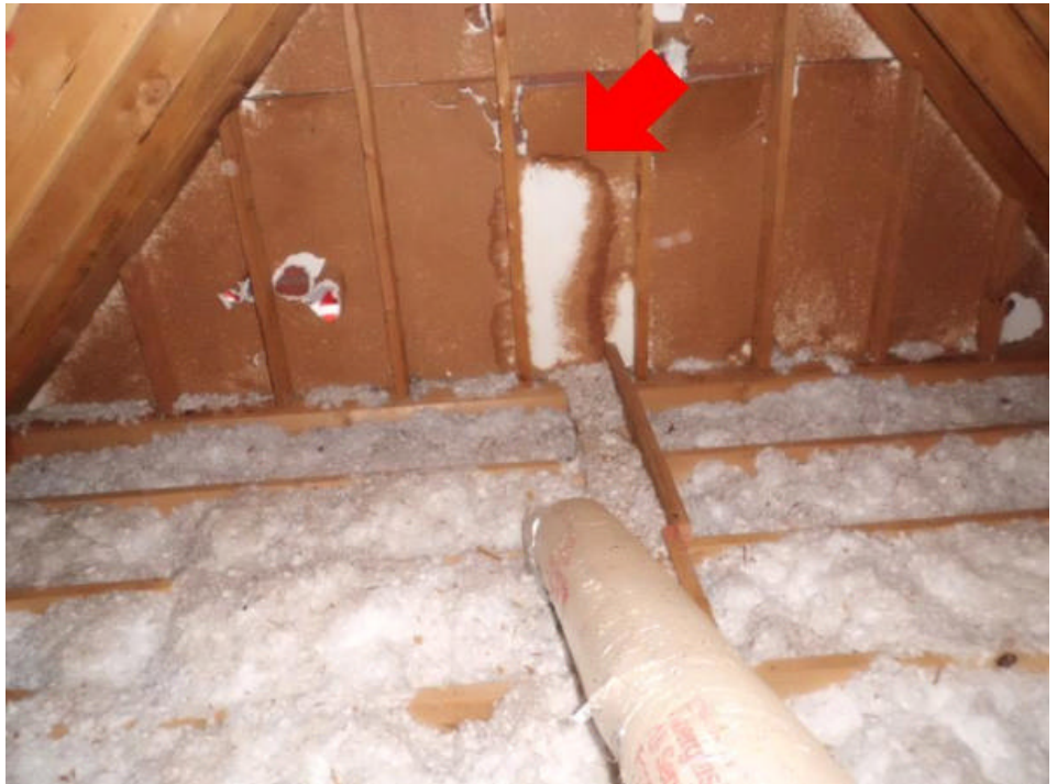
The front gable ends have water staining on the wall sheathing in the attic. The areas were dry at the time of inspection. Recommend monitoring these areas. If water is found to be entering the wall repair will be needed.
