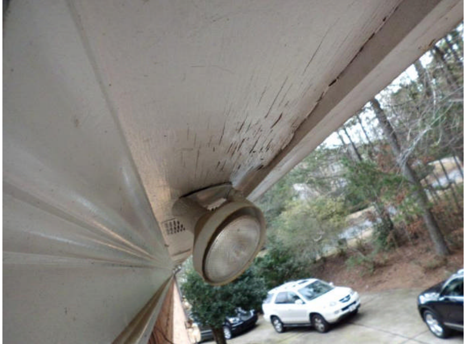
Several soffits around the house are water damaged. Recommend having water damaged repaired.
