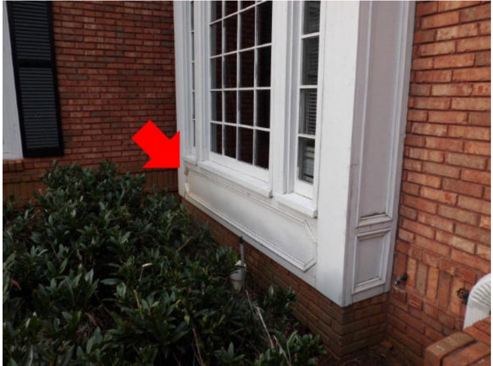
The front dining room bay wall trim and siding are water damaged. Recommend repairing water damage as needed.
