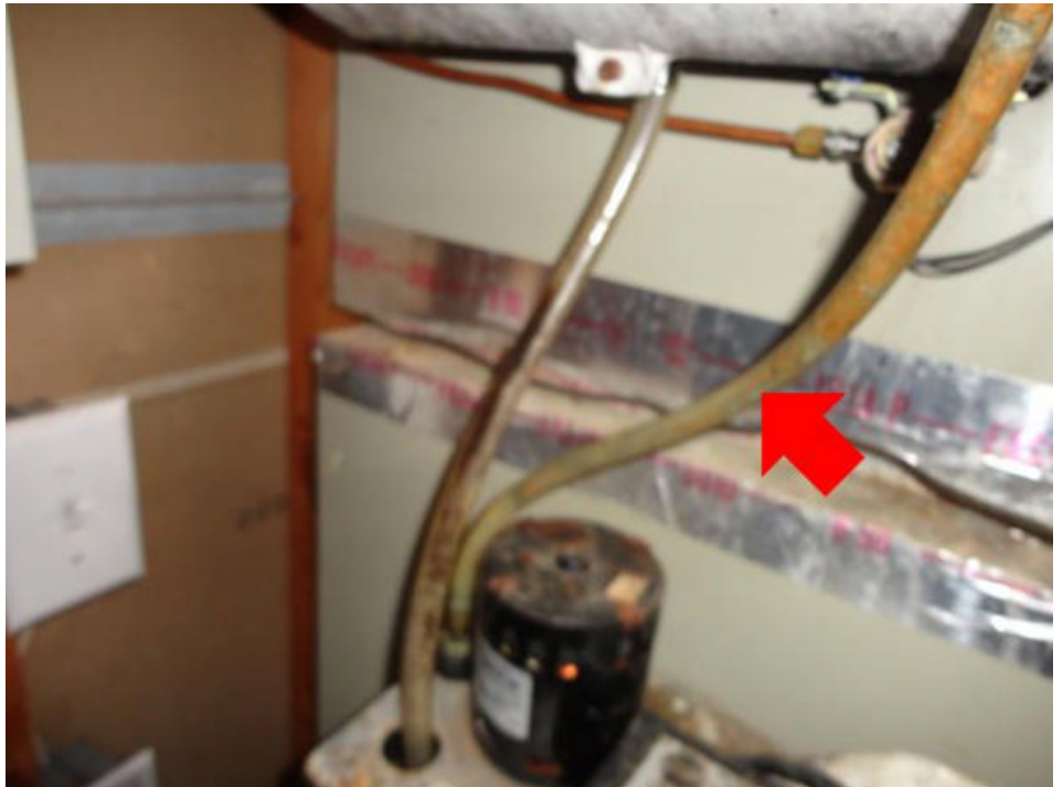
There is a condensate pump installed to remove the water from the furnace cabinet. There is also a humidifier mounted on the system. These are prone to mold and fungal growth. The condensate pump drain tube is dirty. Mildew and scaling occur inside of this line. Recommend cleaning pump tray, line and humidifier with a mild solution of bleach
