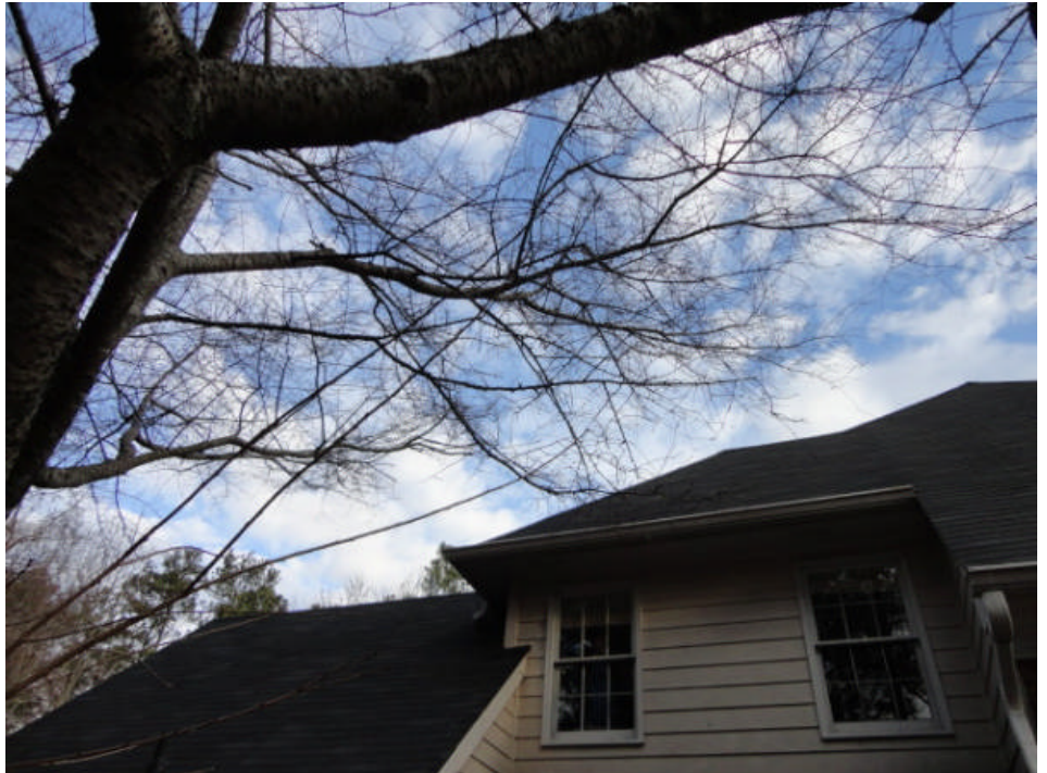
The trees near or overhanging the house need to be trimmed for safety. The dogwood in the front left yard is dead. Recommend removal.
