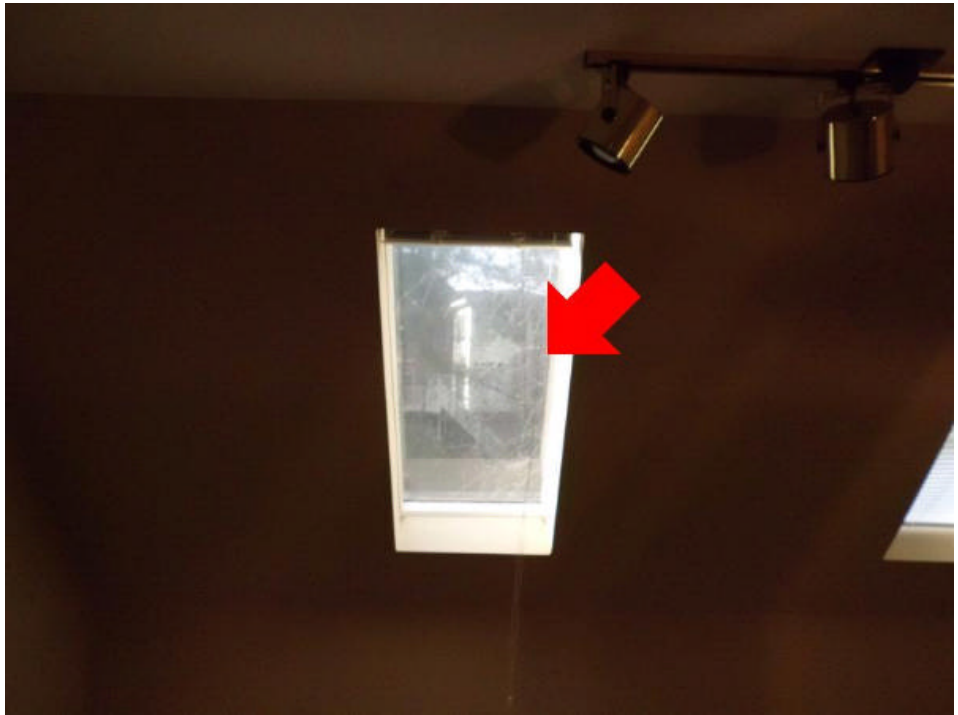
The seals between the glass in the skylights have failed. Recommend replacement of glass in skylights.
