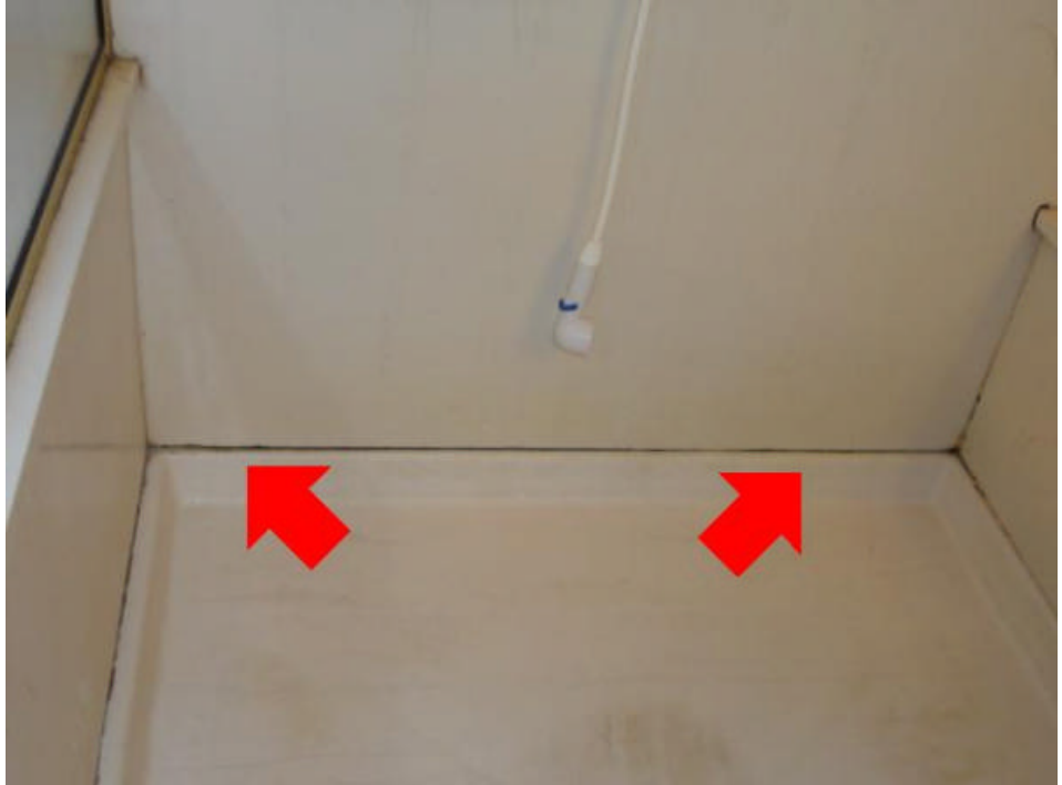
The wall at the shower seam needs to be caulked to prevent moisture from entering the wall.
