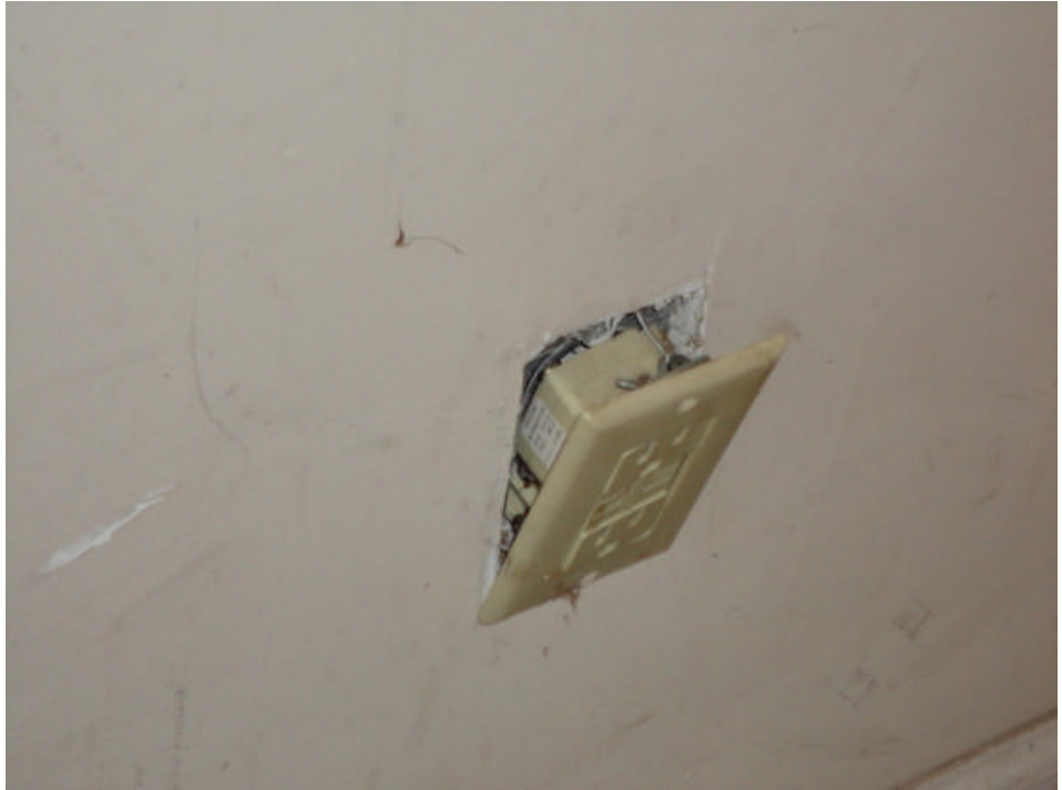
The outlets in the garage are loose and not properly secured inside of their mounting boxes. Recommend repair.
