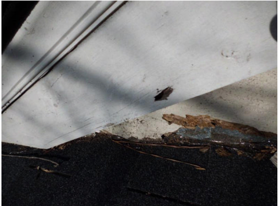
Several fascia boards around the house are water damaged. Recommend repairing water damage.
