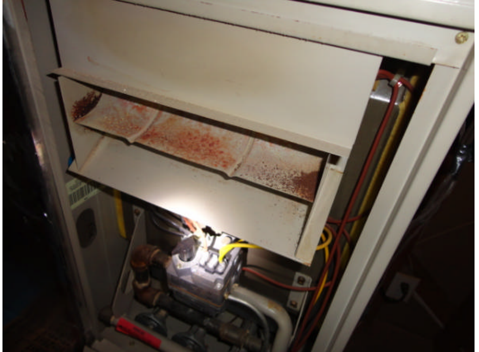
There is evidence of rust in or around the central unit. Recommend a trained HVAC technician inspect and repair or replace as needed.
