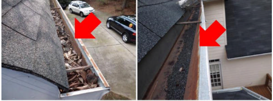
The gutters and downspouts are clogged and rusting. Several gutters are coming loose. Recommend securing and cleaning gutters. The rusting should be sanded and painted.
