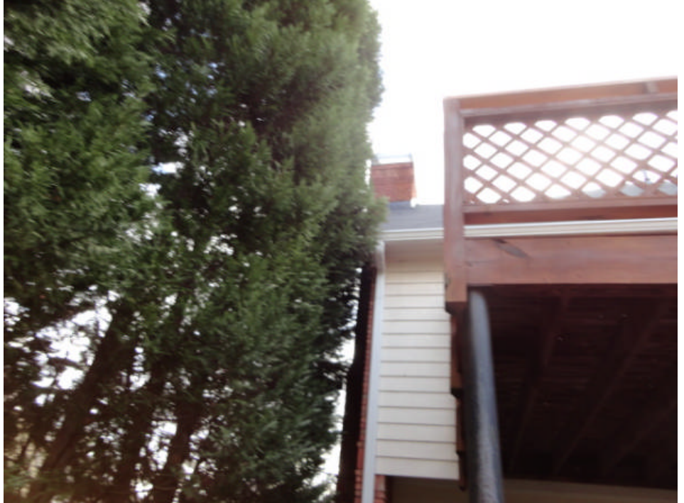
The bushes need to be trimmed so that there is good airflow between the bushes and the building structure. This will help prevent water damage.
