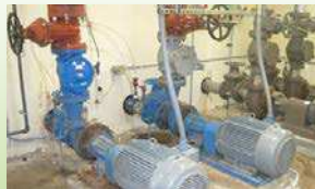
Booster Stations and Other Pumps
