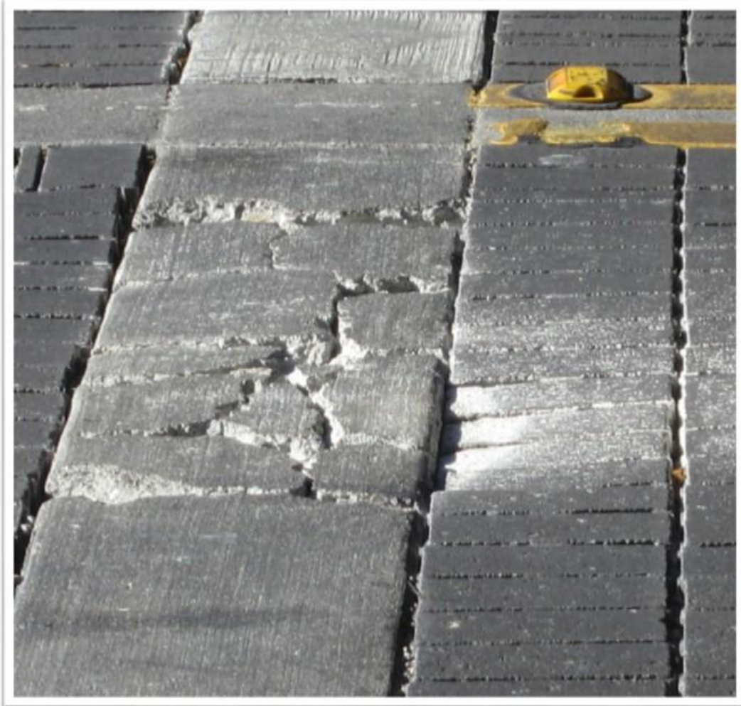
Section of concrete on Castillo Street which will undergo repairs.
