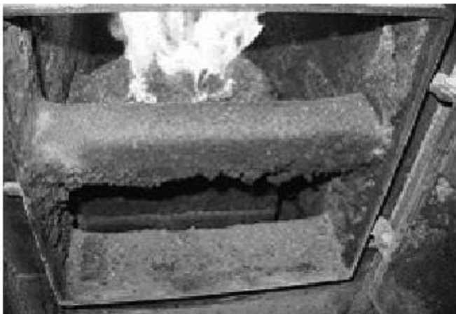
Fig. 13 Very dirty combustion chamber.
