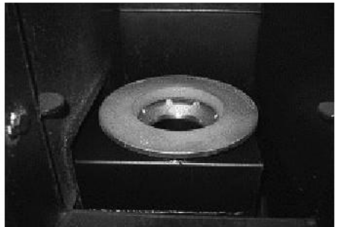
Fig. 14 Very clean combustion chamber.
