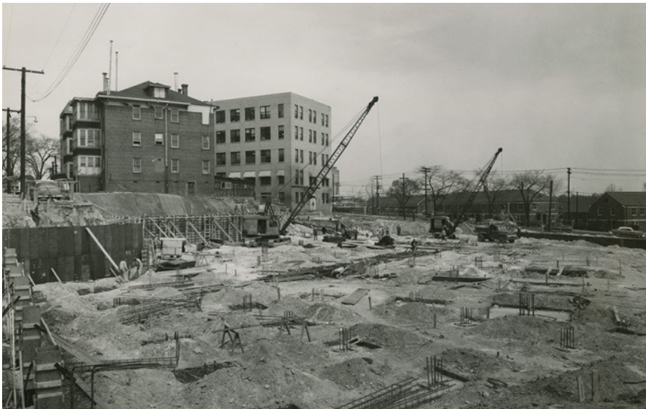
1955 addition to the Highway Department building. The original 1930s building is in the center.
