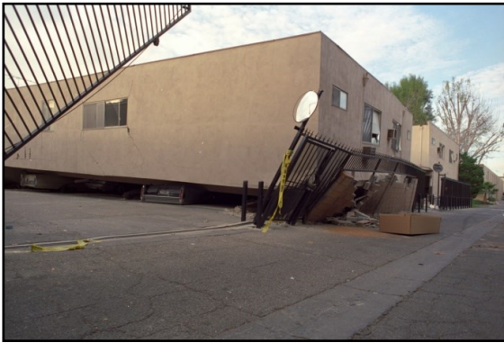
Above: Collapsed apartment building after the Northridge Earthquake of January 17, 1994. Image: Gary B. Edstrom, released to public domain.
