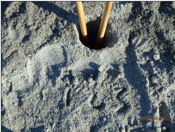
Photo 11. The quantity of rocks within the hole at the center of the constructed berm at Sta. 676+00 between 0-1 feet below existing grade was 3, between 1-2 feet was 4 and between 2-3 feet was 2.
