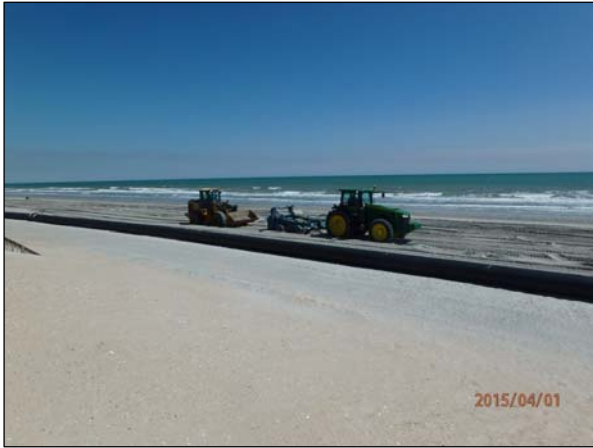
Photo 15. Tigerhole Landscaping commenced rock picking operations up to 36 inches below the constructed grade of the berm area between Sta. 720+00 and 715+00.
