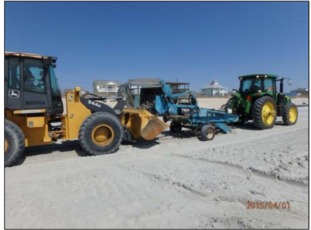
Photo 16. Tigerhole Landscaping emptying the rock picker hopper into a front end loader for removal.
