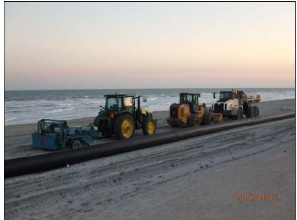
Photo 18. Tigerhole Landscaping's equipment being stored overnight near the shore pipeline in the vicinity of Sta. 720+00.
