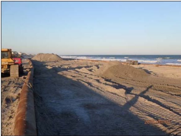
Photo 9. View of the material from the rock boxes being stockpiled seaward of the landward shore pipeline near Sta. 680+00 and 677+00, looking north.
