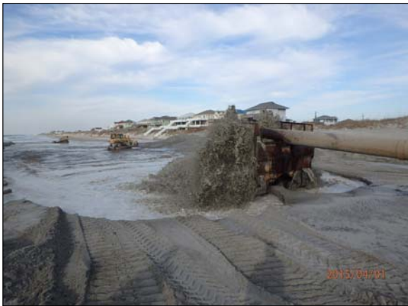
Photo 1. View of the seaward outfall and rock box at 08:50 near Sta. 674+00, looking south.
