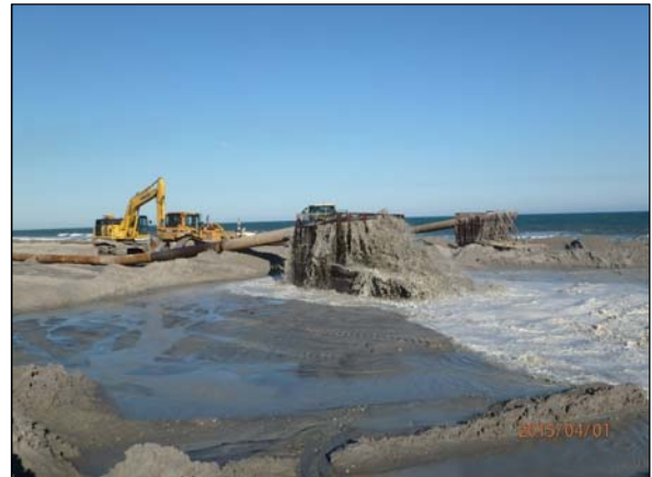
Photo 2. View of the landward and seaward outfalls and rock boxes at 17:45 near Sta. 674+00, looking northeast.
