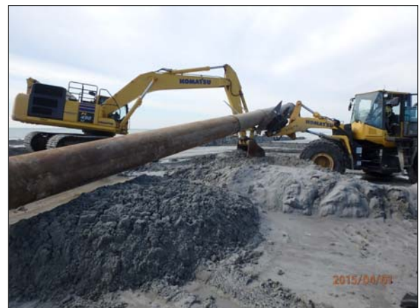
Photo 8. An excavator being used to collect the material from the rock boxes within the discharge area.
