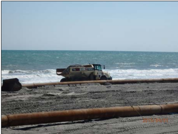
Photo 17. The Town's off-road truck was utilized to relocate 3 truck loads of rock (36 cy) that were removed by Tigerhole Landscaping's rock picker from the constructed berm area between Sta. 720+00 and 715+00.
