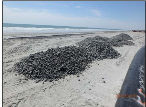
Photo 10. View of the rocks previously collected by the rock picker being stockpiled seaward of the shore pipeline near Sta. 694+00.
