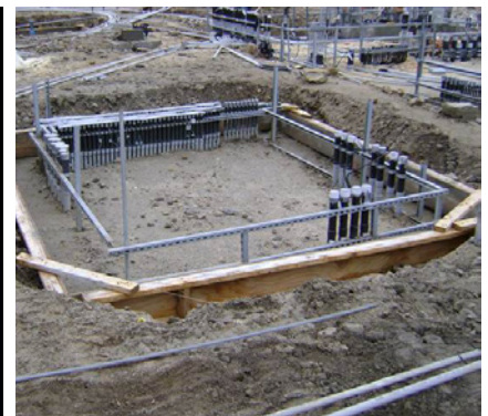
2013 Commercial Award of Excellence in Electrical Construction Winner Hazelton Correctional Facility by Northern Electric
