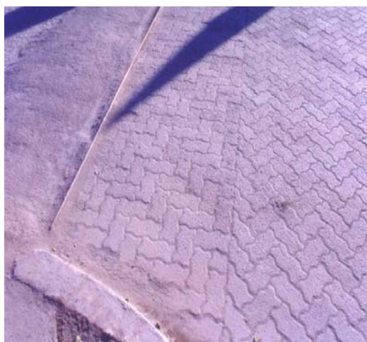
Figure 6. Eroded transition zone.
