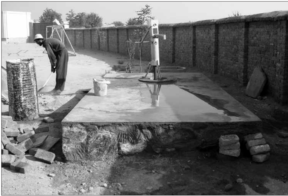
New water well and pump while under construction in Afghanistan. A plaque at the site thanks students at St. Raphael Elementary School in San Rafael for the new resource.
