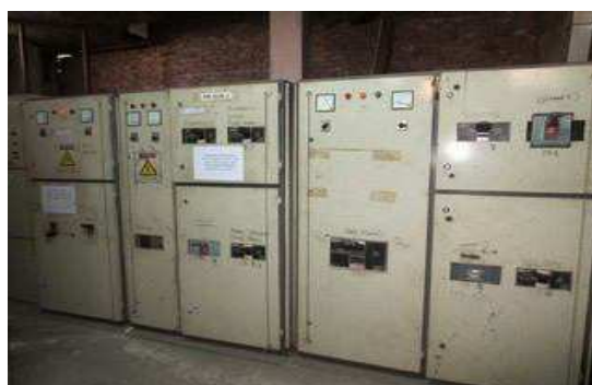
Figure 9.7: Low Tension Panel [2].
