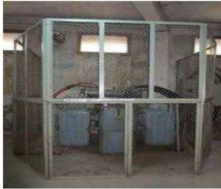
Figure 9.2: Step down Transformer [2].
