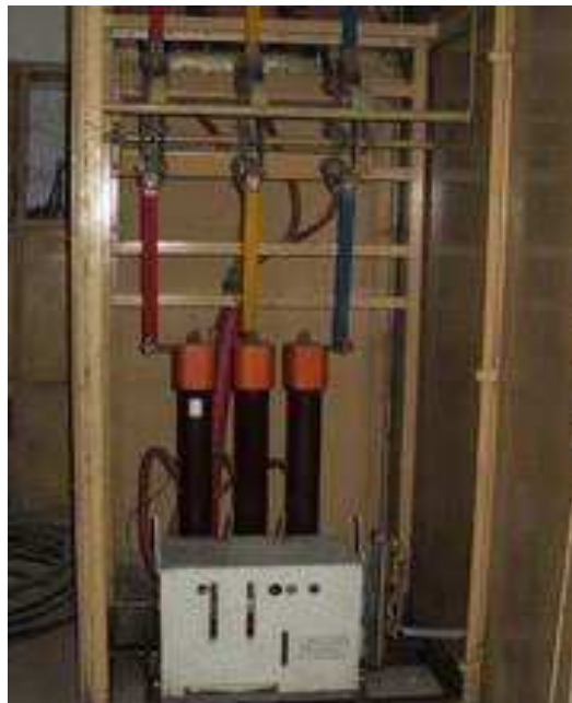
Figure 9.1: High Tension Panel [2].
