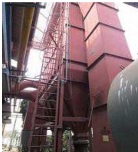
Figure 7.11: Air blower, Fume blower, Filter Bag house and Dust Filter [2].
