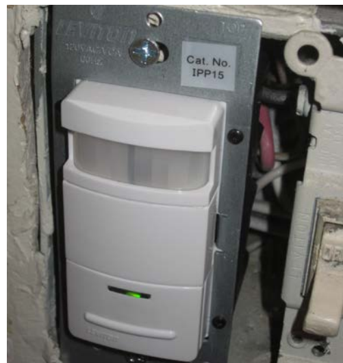
Lighting controls, like this occupancy sensor, helped to automate control and reduce energy consumption.
