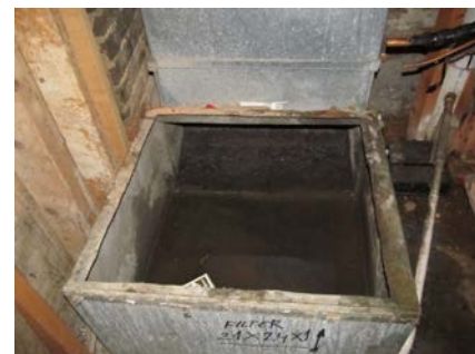
The existing plenum had 4" of standing water from an improperly plumbed condensate line! Replacing and re-plumbing saved energy and improved indoor air quality.
