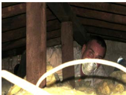
Air sealing at the Sasha Bruce group home in Washington DC required accessing some tight spaces.
