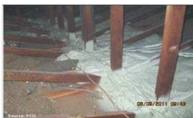
Application of membrane and sprayfoam to seal ductwork and air leakage pathway
