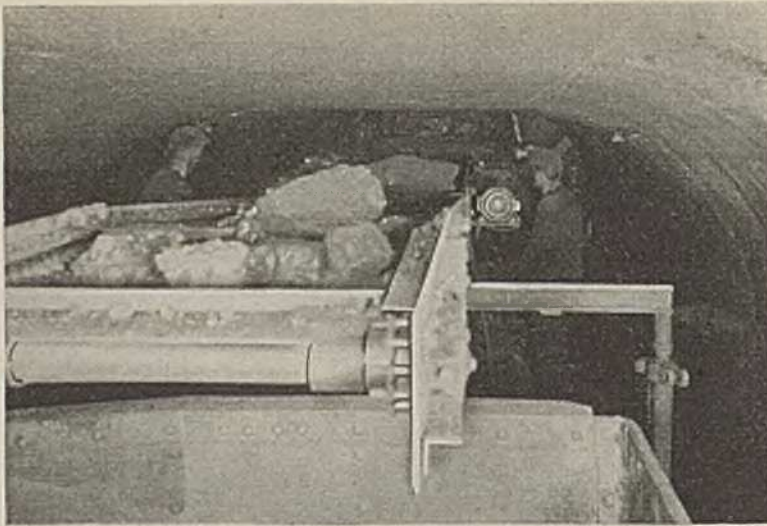
Close-up of the Machine in Operating Position. About 51 Per Cent of the Coal Produced by This Machine Is Larger Than 2 In.
