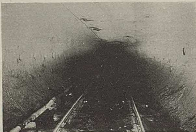
This Method Assures Straight, Smooth Ribs and Arches Which Generally Hold the Roof Secure Without Timbers.
