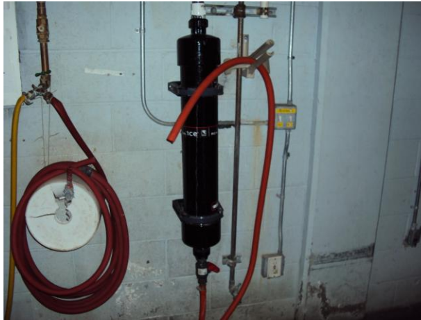
FIGURE 4. INSTALLED REALICE SYSTEM
