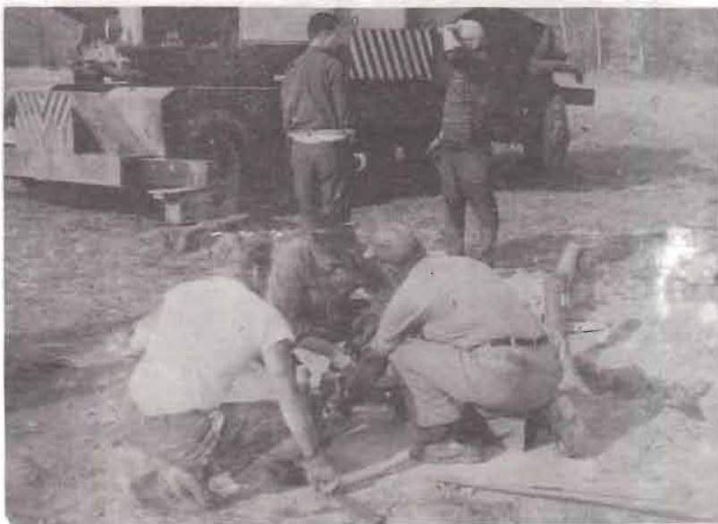
Workmen check alignment of the base bolts before first mast is raised.
