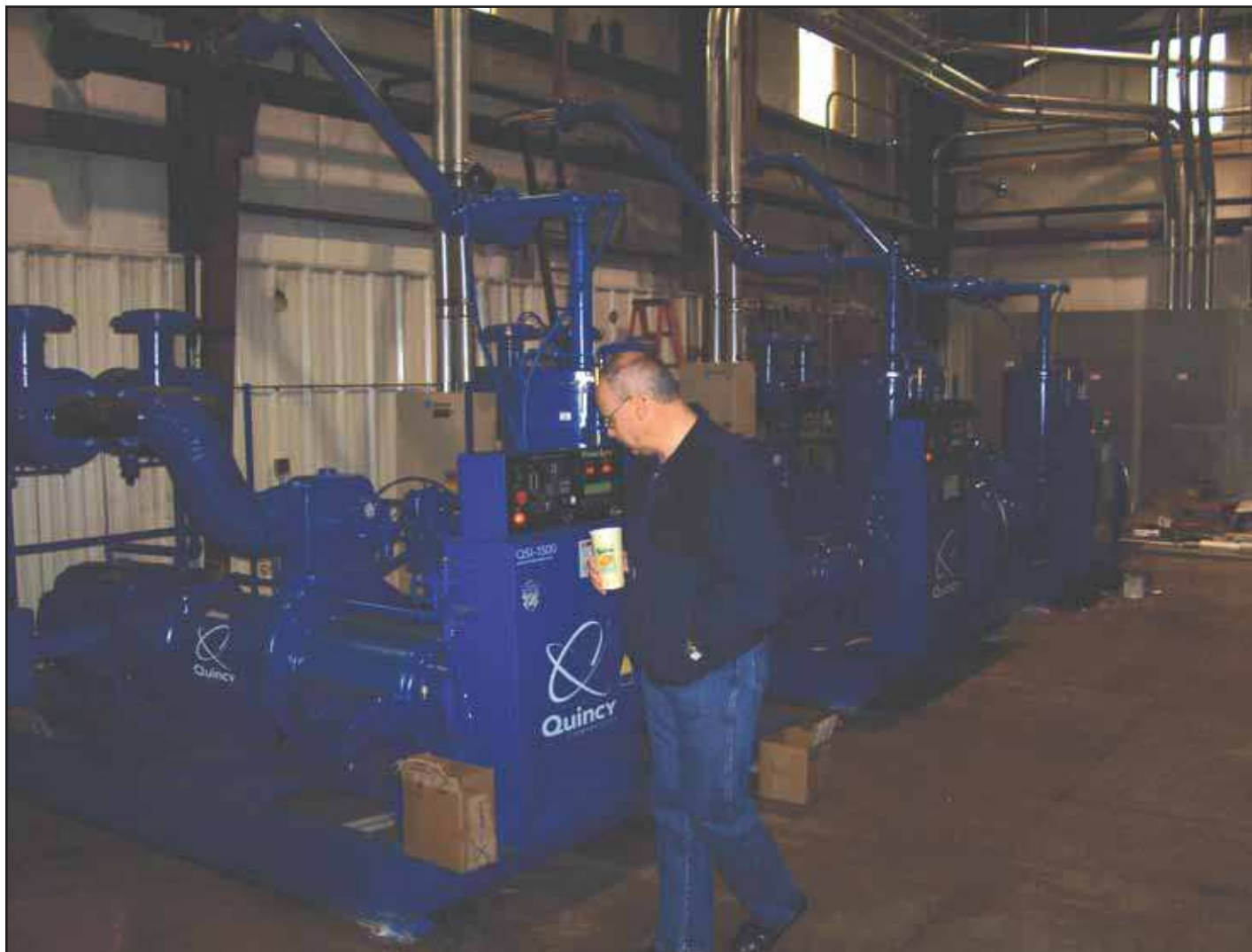
Steel Forging Facility in Michigan with Brehob/Quincy Rotary Screw Compressors
