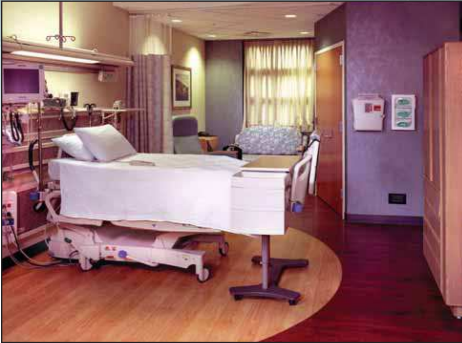
Medical compressed air systems are often used in intensive care units. Dan Francis, Mardan Photography
