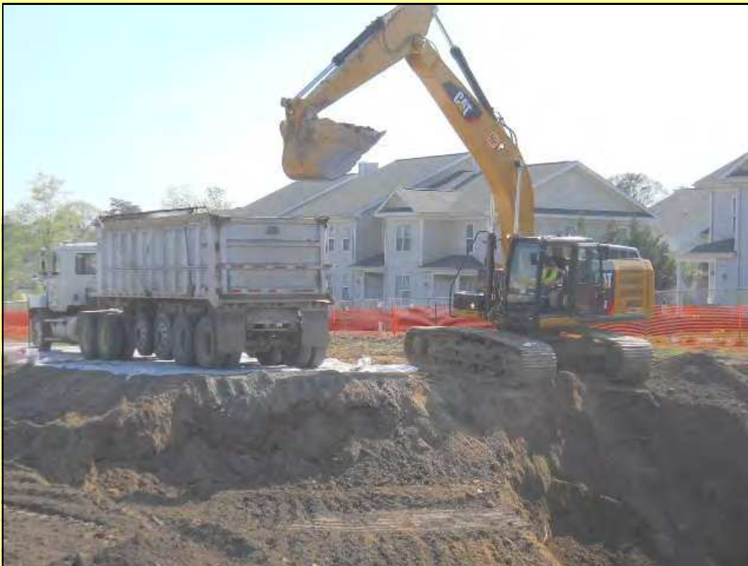
Photo of the site during the excavation of the approximately 30,000 tons of waste.
