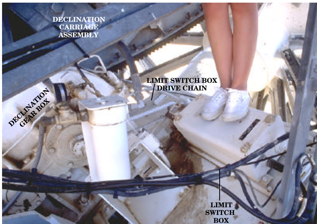
DECLINATION LIMIT SWITCH BOX
