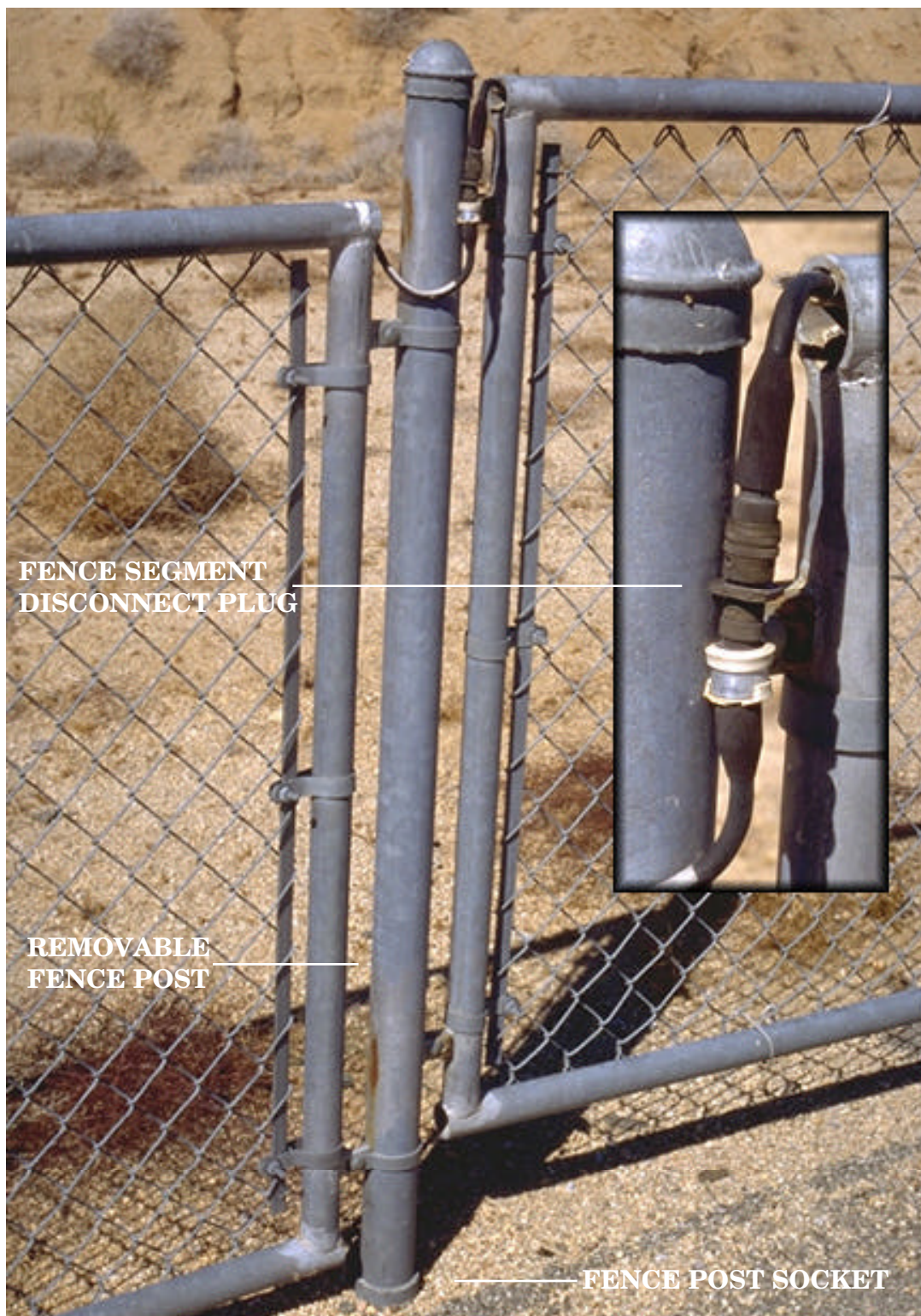
GAVRT ANTENNA PERIMETER INTEGRITY FENCE
