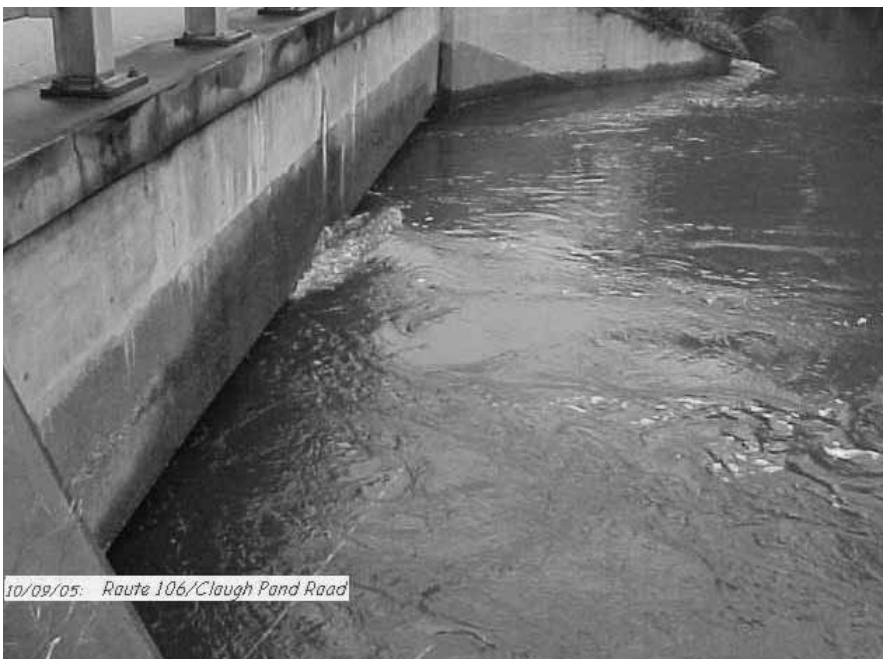
Shaker Brook going under the bridge at Route 106/Clough Pond Rd. intersection.
