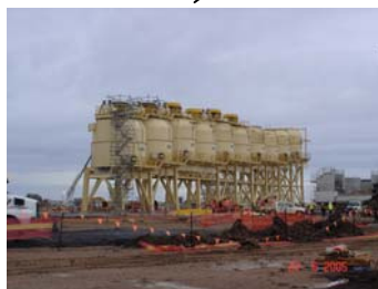
Plate 4: Flotation tanks – process plant
