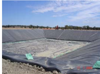
Plate 2: Contained Water Storage D6 – HDPE lined.
