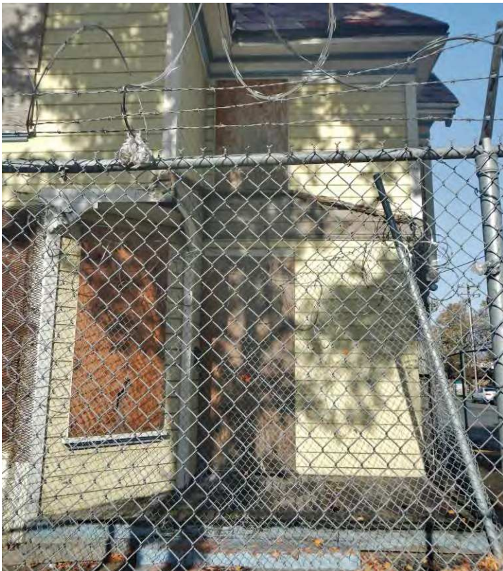
Missing front porch, viewed facing north.
