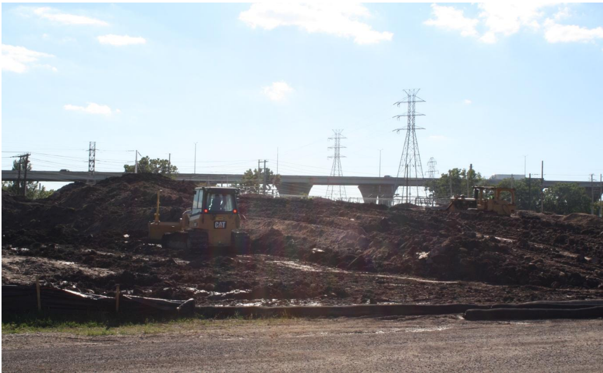
Excavated material stockpile for reuse on Contract 34 Digestion and Solids Facility and Contract 35 Demolition of existing solids building and site work.
