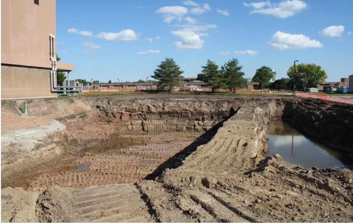
Solids Facility excavation looking east. Electrical duct bank running down middle of excavation to be removed later.
