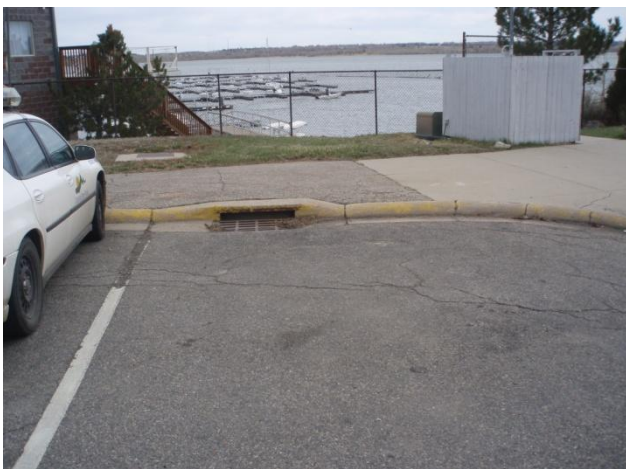
Photo 2 Inlet w/ Direct Reservoir Connection
