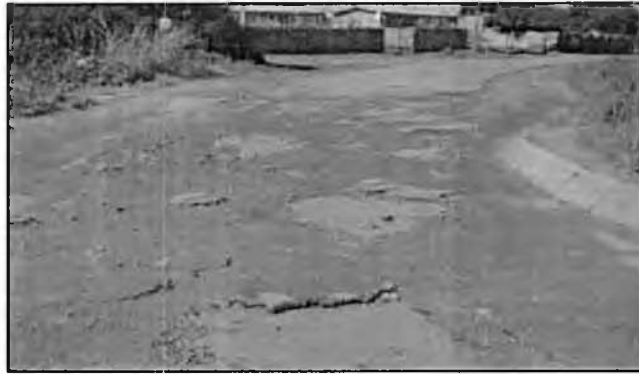
Fig. 4 State of the road at Ziyambi Drive and Matongo Way intersection in Senka-Nehosho area.
