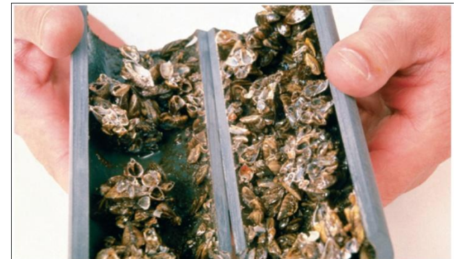
(a) Clogging a pipe
