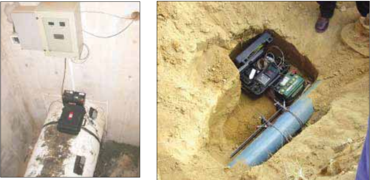
Figure C-1: Initial logging of flows with temporary clamp-on ultrasonic meters on large and small diameter pipes
