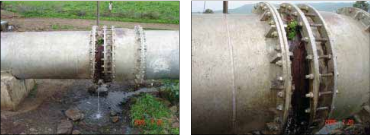
Figure B-1: One of the leaking joints on the Narmada Pipeline
