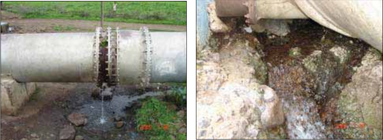
Figure 10: Visible leaks on 1200 mm Trunk Main from Narmada
