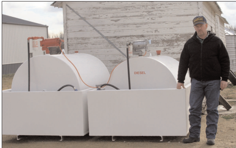
Chris Visser's leaking fuel tank on his farm was located within 100 yards of the family water well. He replaced the faulty tank and installed containment tanks beneath them.
