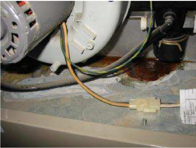
Condensate leaking inside basement furnace.
