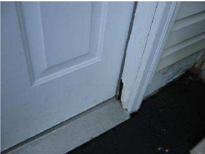
Rotted trim at door to garage.
