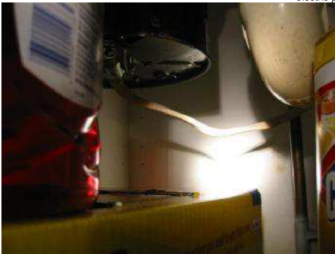
Unprotected electric cable below kitchen sink.
