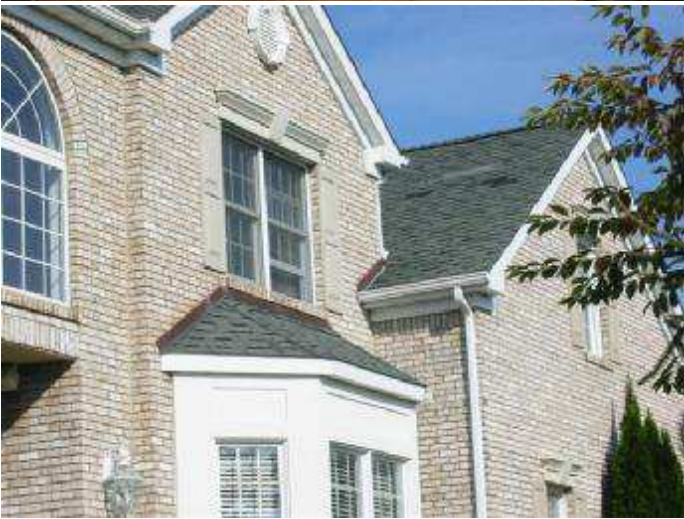
Damaged, missing roof shingles above garage area.
