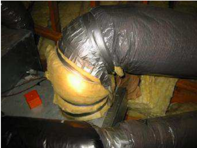
Damaged wrapping on insulation in attic. Peeling duct tape. Sample of kinked ductwork in attic area. Contact a heating system contractor.
