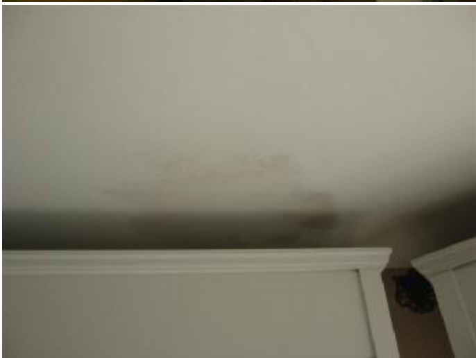
Moisture stains at office room ceiling. Contact a plumber.
