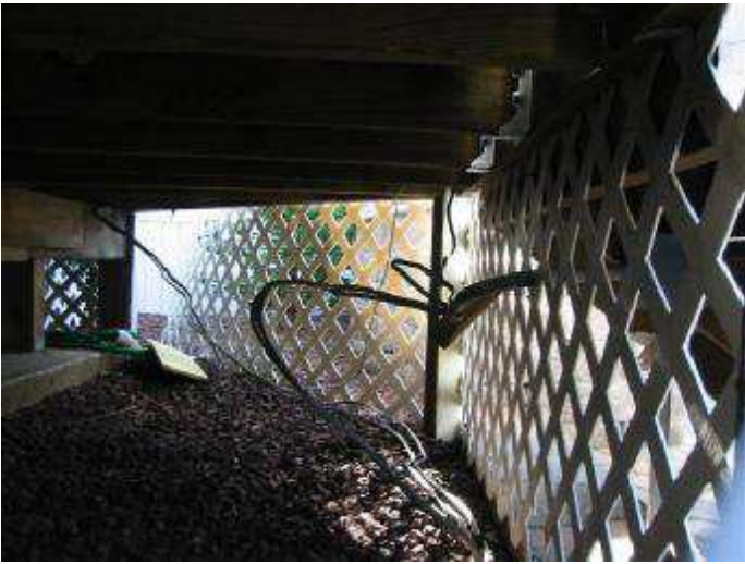
Dangling electrical cable near hot tub.
