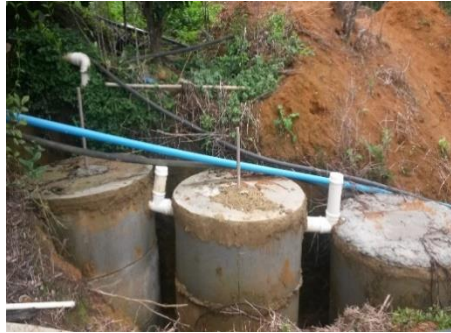
Figure 15: Biodigester septic tank in Barracão dos Mendes (Image taken by the author)
