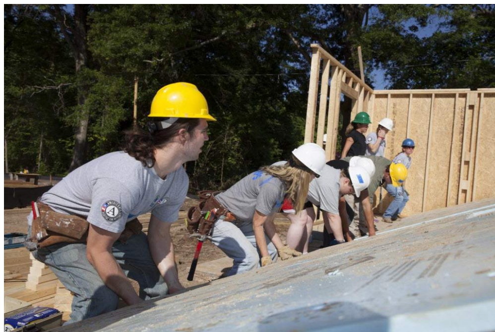
Pittsburgh AmeriCorps Member, Andrew Dadig, works with fellow AmeriCorps members from across the country to raise a wall on a housing project in Raleigh, North Carolina in 2014.
