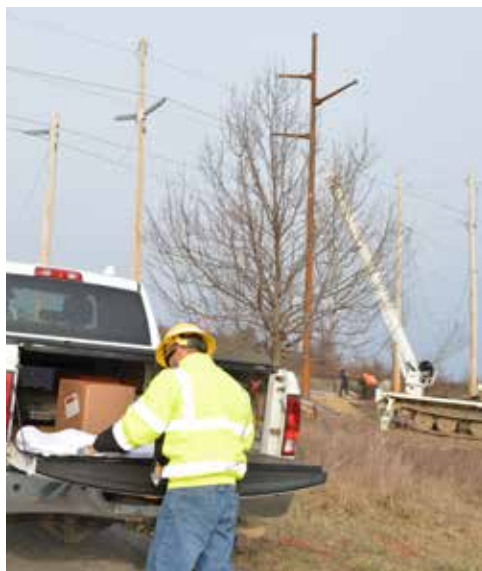
Line Foreman Chris Calogero reviews the Environmental Management and Construction Plan on the C-Line upgrade while work continues in the background on Frost Hill Road in Pleasant Valley.
