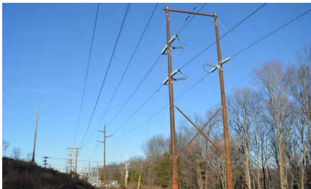
A portion of the upgraded A-Line leading into the Todd Hill substation. The new design consists of single and two-pole steel Corten structures, which have a brown patina to help blend in with landscape. There will be 112 structures and 139 poles.
