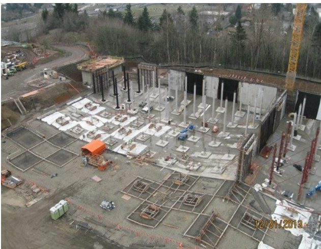
Aerial photograph of 25 million gallon buried water reservoir Andrew helped design and provide engineering services during construction for the Portland Water Bureau.
