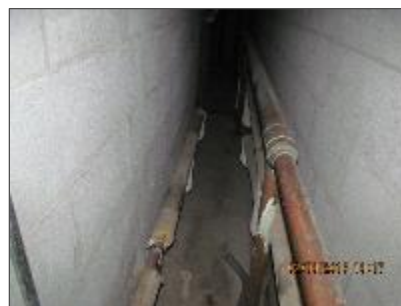
Photo 4 – Damaged parging cement insulation in Pipe Chase P02. Parging cement debris present on the floor.
