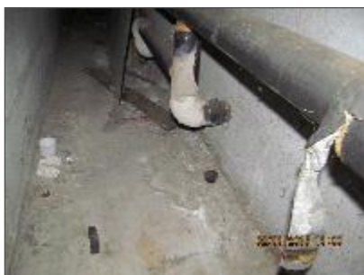
Photo 3 – Damaged parging cement insulation in Pipe Chase P01. Parging cement debris present on the floor.
