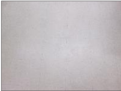
Photo 19 – Typical view of asbestos-containing floor tile both exposed and concealed beneath millwork in classrooms.
