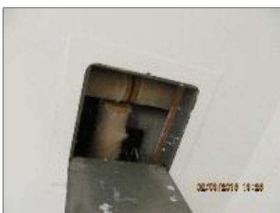
Photo 7 – Parging cement on domestic water pipes above ceiling in Washroom 102A.
