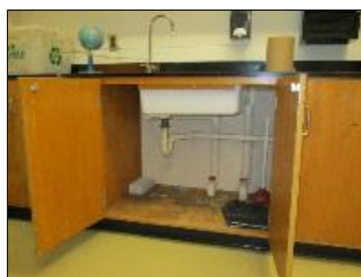
Photo 8 – Parging cement on domestic water piping beneath a sink on the 2 nd floor.
