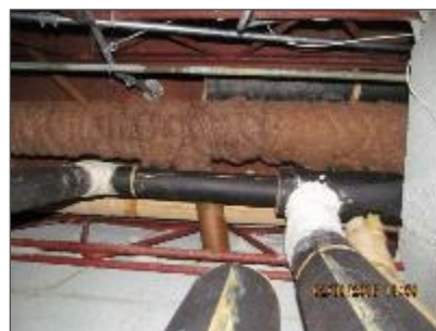
Photo 2 – Unjacketed parging cement on an unknown pipe system in Pipe Chase P01.
