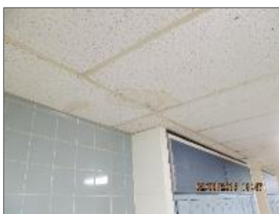
Photo 9 – Non-asbestos ceiling tile in Corridor 108H.
