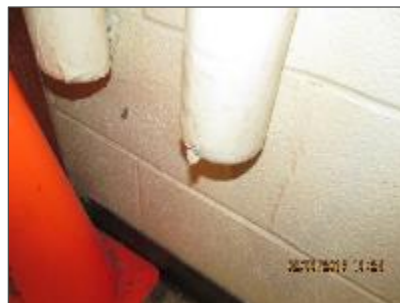
Photo 6 – Damaged butt ends of insulation in Custodian 100B.
