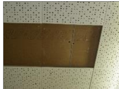
Photo 15 – Gypsum panels supporting ceiling tile with no mud on seams in a typical classroom.
