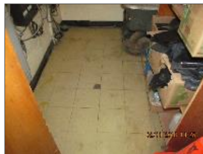
Photo 18 – Asbestos floor tile in Custodian 100B.
