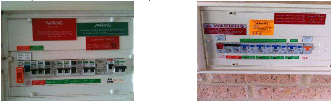
P-13: Main switchboard / meter panel and upstream switchboard labeling (One or more pictures to cover all labels below)
