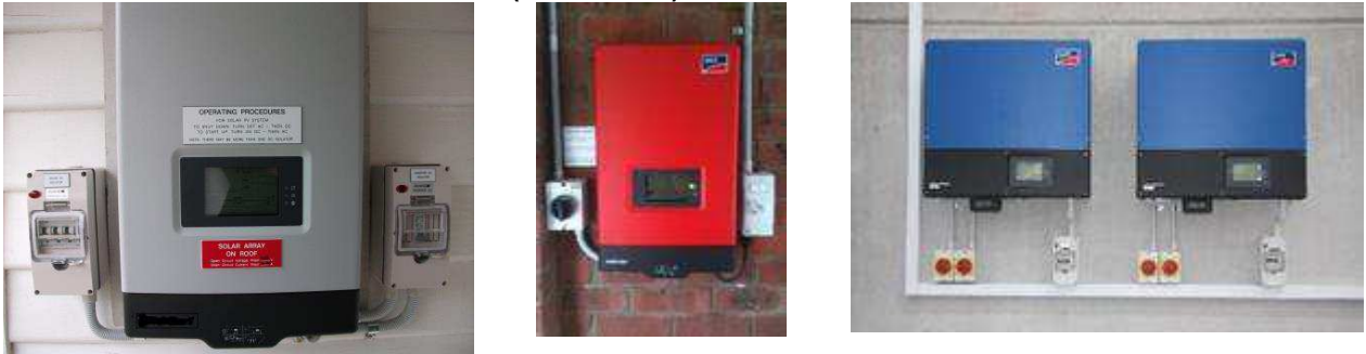
P-11: Inverter and isolators installed (broad view)
