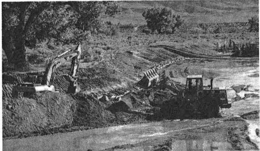
Heavy equipment works on a Dayton Valley Conservation District river bank stabilization project in the Carson River along River Road this fall. HANDOUT
