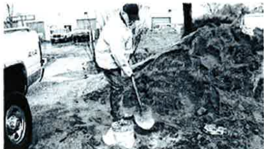
Steve Young shovels dirt to make sandbags on Friday to prepare for flooding at his North Edison Way business. BRIAN DUGGAN/RGJ
