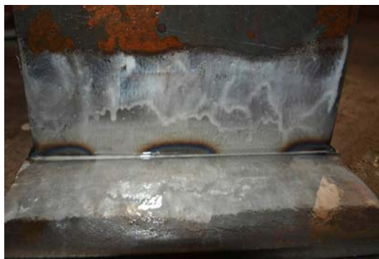
Fig. 9. Elements with the excessive amount of the anti-spatter substance applied in the joint interface
