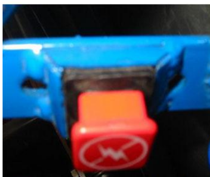
The welded metal tabs constraining the switch
