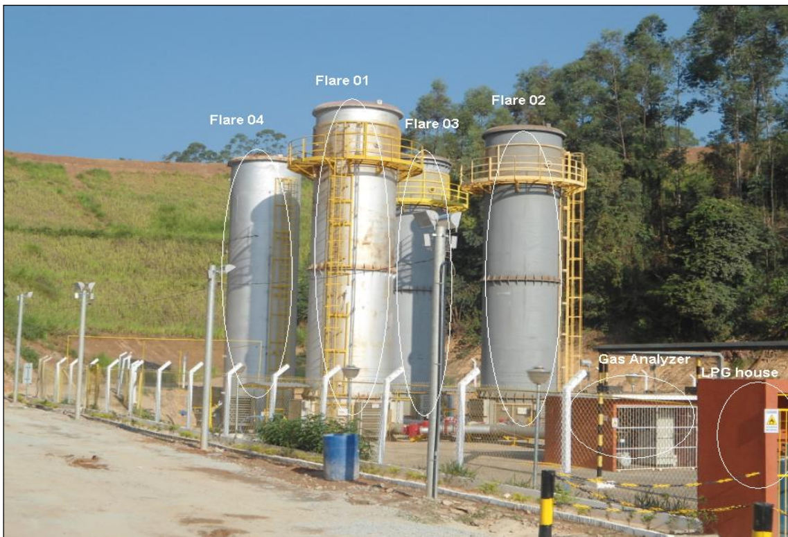
Figure 2 – Partial view of the project’s LFG destruction plant (picture dated January 2012).
