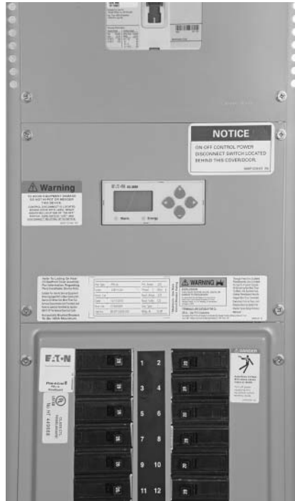
IQ 35M mounted and wired in Eaton panelboard. Closeup photo showing IQ 35M panelboard integration and deadfront cover.
