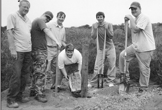
Eagle Scout candidate Erik Johnson (pouring concrete around post) and his crew built a fence at the 17th Street entrance to the Elfin Forest. The crew (L-R) included Troop 345 Scoutmaster Bill Holden, Brandon Pettis, Erik's father, Erik, Aaron Marley, and John Mastin. Photo by Pat Sarafian.
