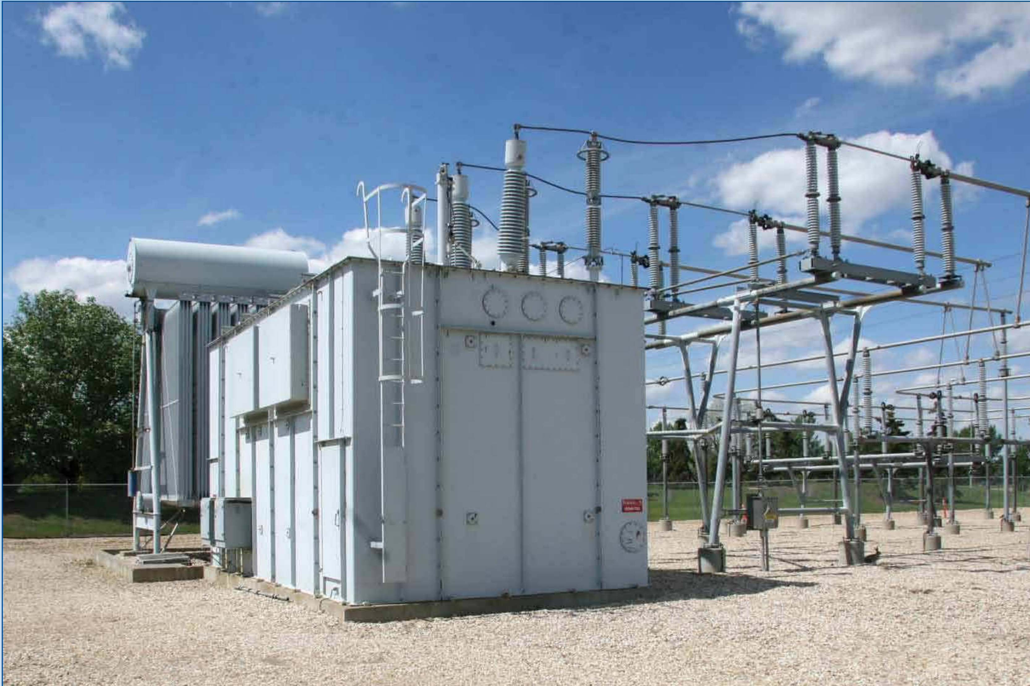
Example of a substation in an Edmonton community – with a transformer and connection equipment.
