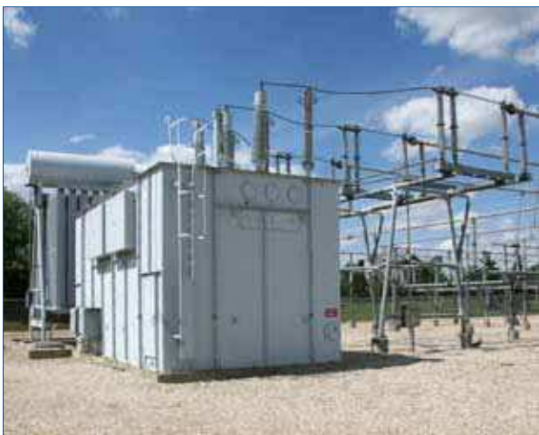
Example of a substation in an Edmonton community – with a transformer and connection equipment.
