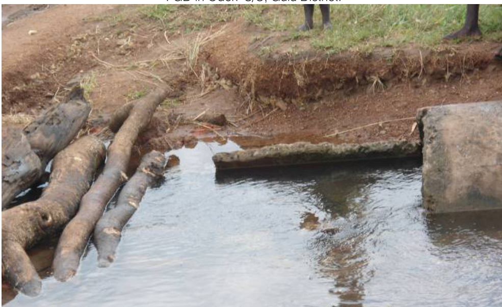
Broken bridge in Odek S/C, Gulu District
