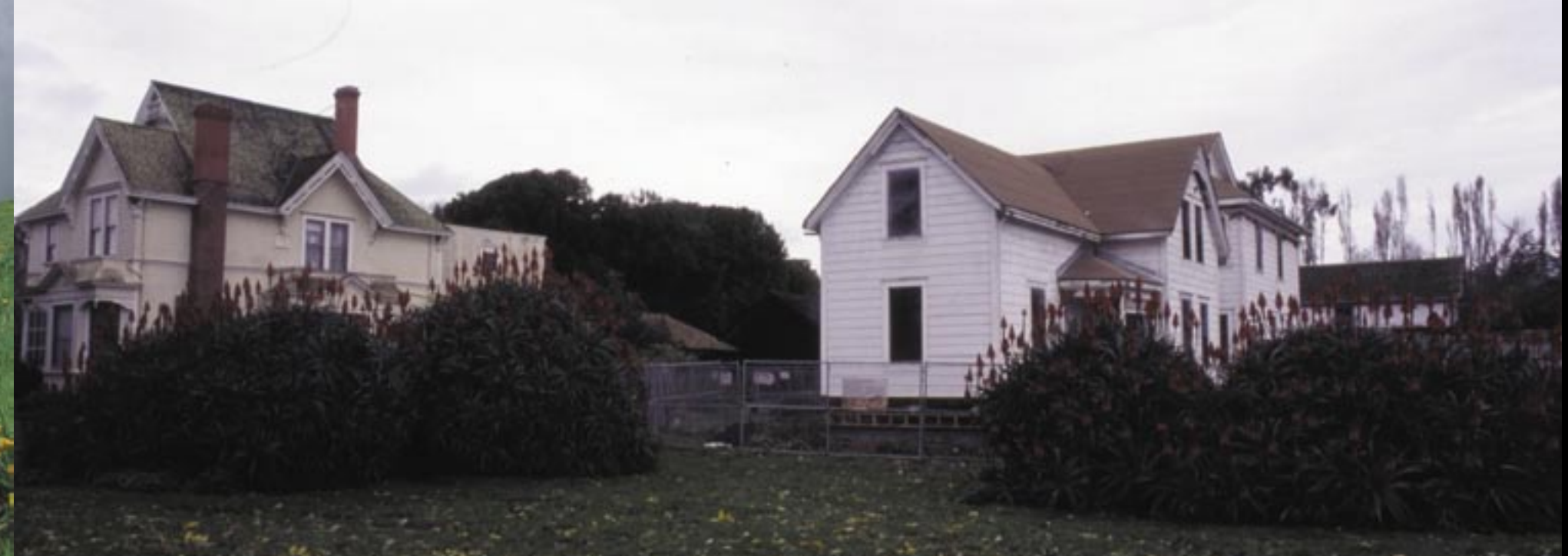
▲ Meder House currently being renovated, pictured next to the Victorian at Wilder Ranch.
