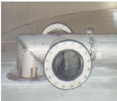
(2) 16" Series 37 as drain valves.
