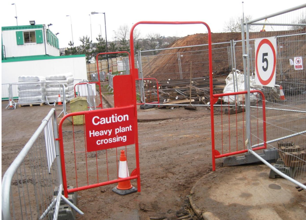
Properly integrated pedestrian crossing point with signage used in conjunction with pedestrian barriers and Heras fencing
