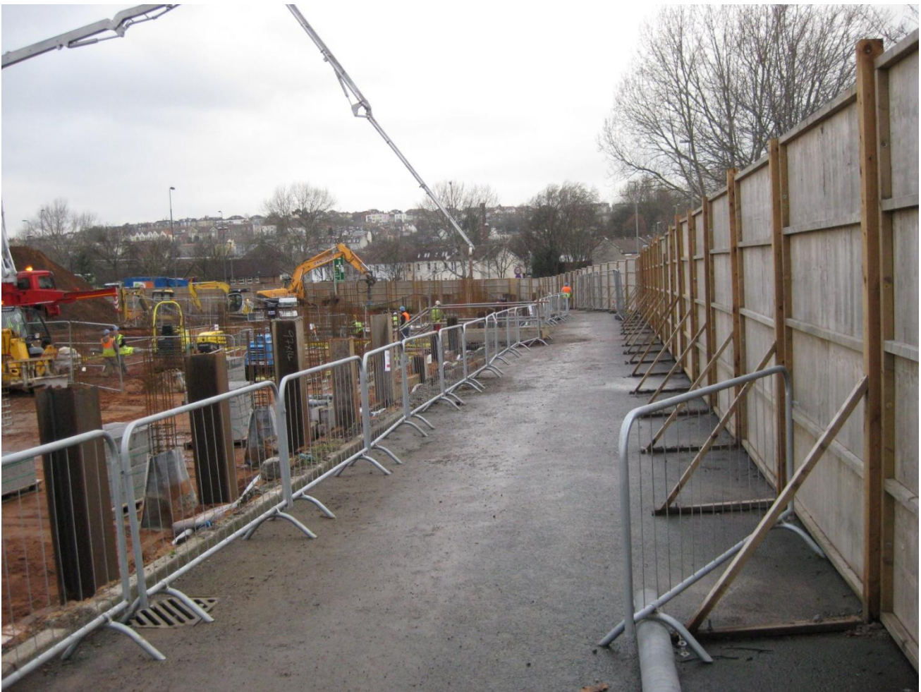
Pedestrian Barriers used to segregate pedestrian access from site activities. Note free standing hoarding to allow for temporary repositioning
