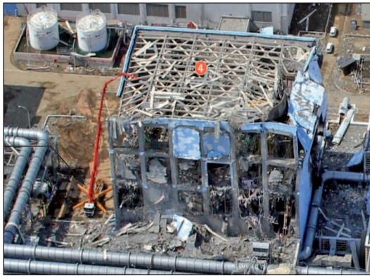
Fig. 8. A mobile concrete pump with a capacity of 120 t/h and a flexible, truck-type arm with a length of 58 m was used for about three hours in the late afternoon of 22 March 2011, to spray a total of 150 tonnes of sea water from the top onto the destroyed unit 4 and to fill the spent fuel cooling pool with water. This measure was repeated several times on the following days
