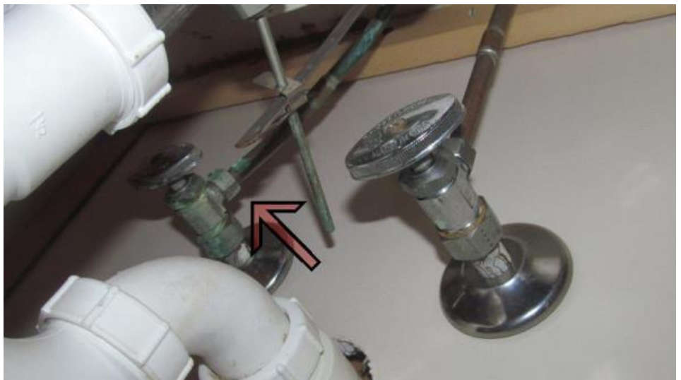
There is evidence of a past leak under the sink. Monitor.
