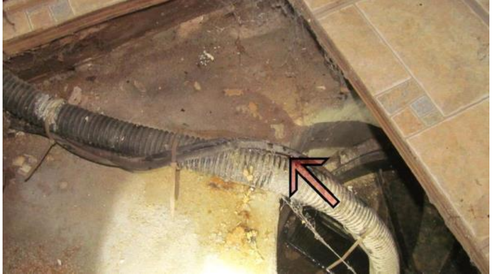
Sump pump condition: Replace the leaking drain hose and seal the crack to deter mold under the floor.
