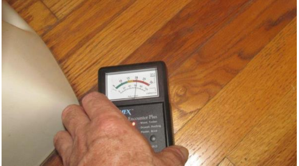
Wood floor stained at the toilet. The wood is damaged. Repair the floor. See toilet for more details.
